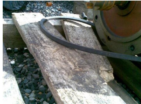
X Broken planks
