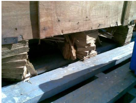
X Poor wood structure
